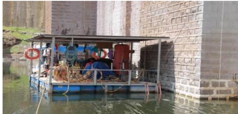
Racking and pointing in upstream face RR Joints at under water at Sholayar Dam
