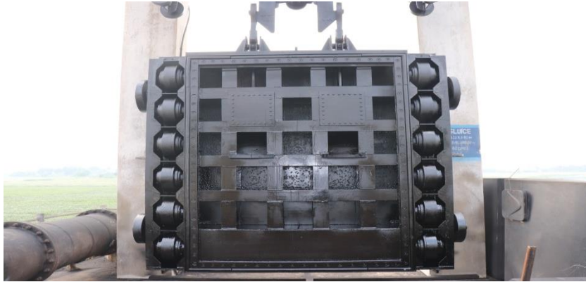
River Sluice Emergency Shutter at Kelavarapalli Dam
